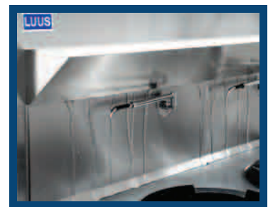
Water Cooling System
